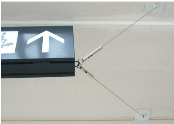
Vibration stopper in station
